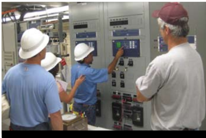
Fig. 6. Resynchronizing the island to the grid using a synchroscope.
